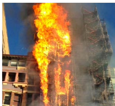
Macquarie St, Sydney. May 2018. No casualties. 20 people evacuated. Scaffolding set up to remove cladding, catches fire.
