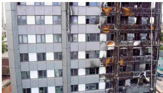
Images after the fire show evidence of melted cladding on the tower’s columns
